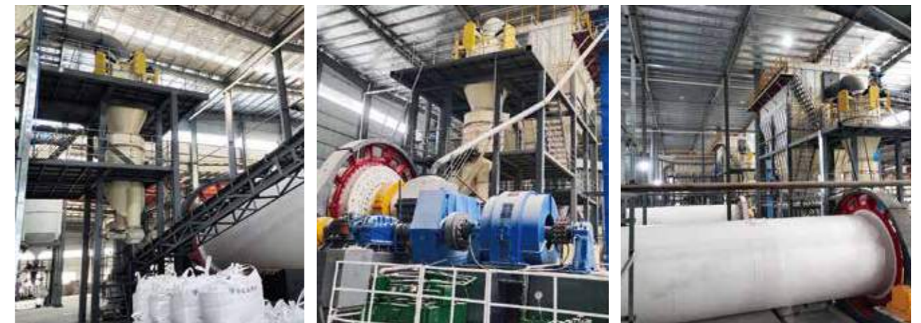
40,000tons/Year Calcium Carbonate Ball Mill Plant and Coating Plant In Egypt, Year 2018 (Φ2.2*5.5m Ball Mill)
