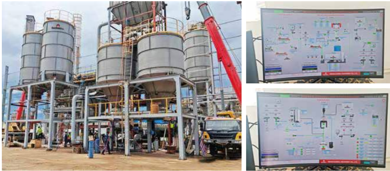
40,000tons/Year Calcium Carbonate Ball Mill Plant and Coating Plant In Tanzania, Year 2025 ( \Phi 2.2 \times 5.5 m ball mill)
