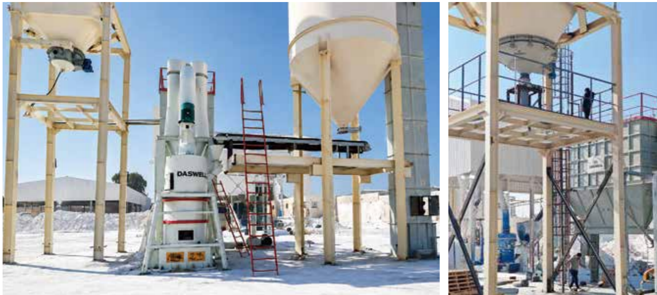
3T/H DR-28 Ring Roller Mill Calcium Carbonate Grinding Plant Expansion Project In Minya, Egypt, Year 2026
