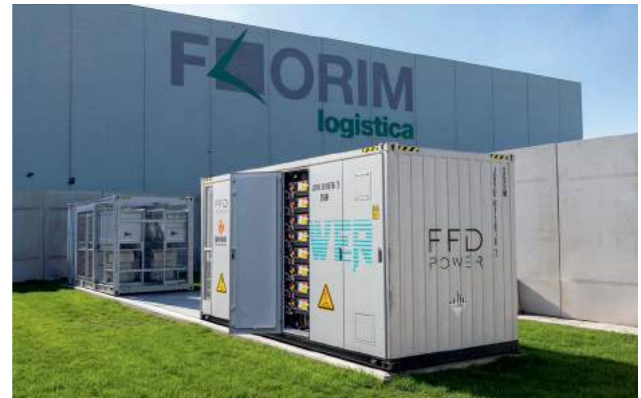
Battery Energy Storage System (BESS) | FLORIM main headquarters (Fiorano Modenese - MO - Italy)
