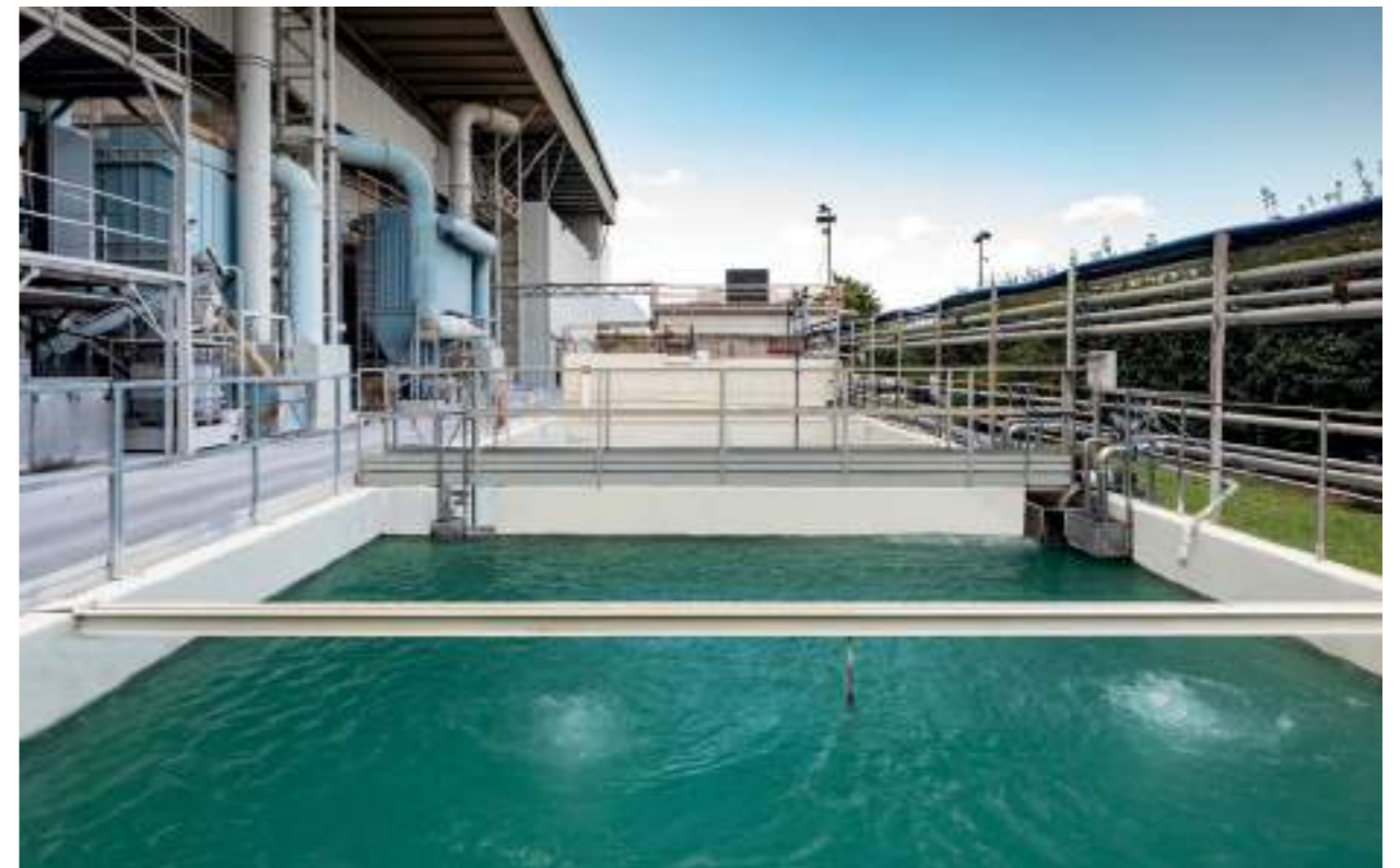
Process wastewater treatment at Florim headquarters (Fiorano Modenese, Modena, Italy)
