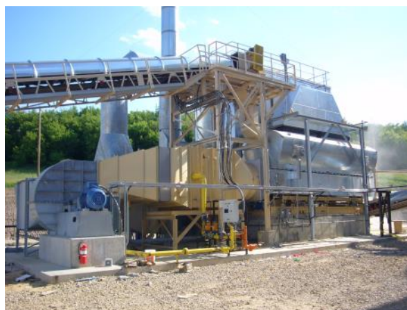
FLUID BED SAND DRYER
