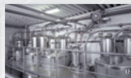
Pneumatic conveying systems
