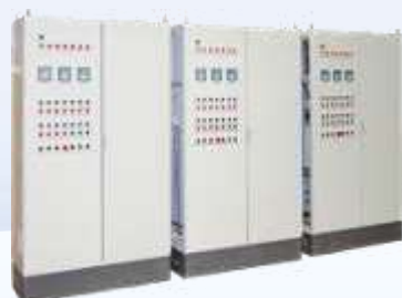
ELECTRICAL CONTROL CABINET AC
