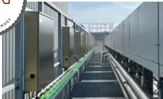
The walkway by the evaporators provides easy service access.
