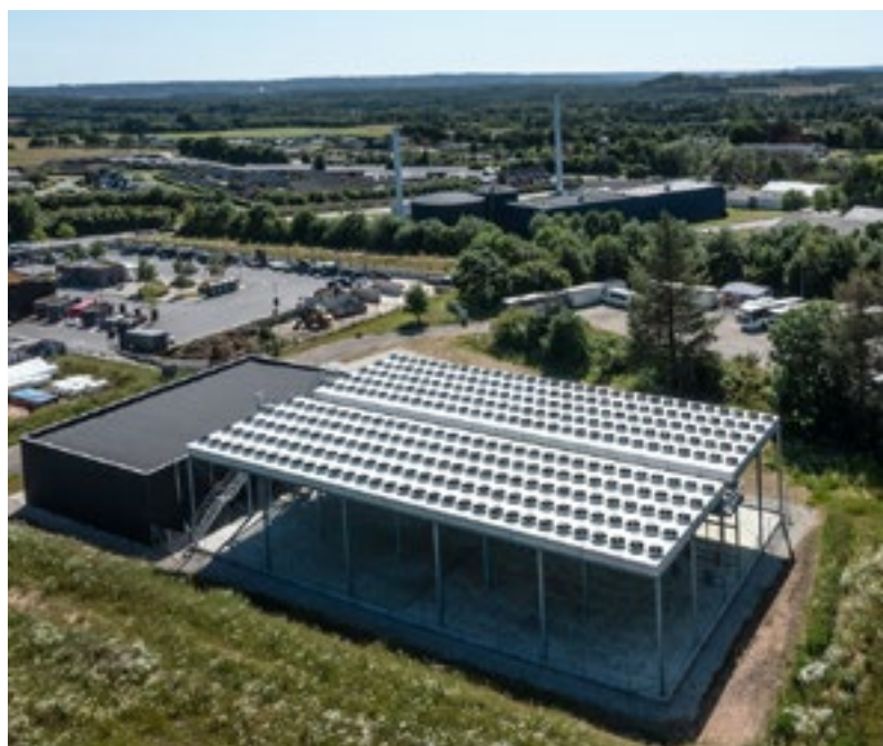
New nearby site with energy collectors and heat pumps
