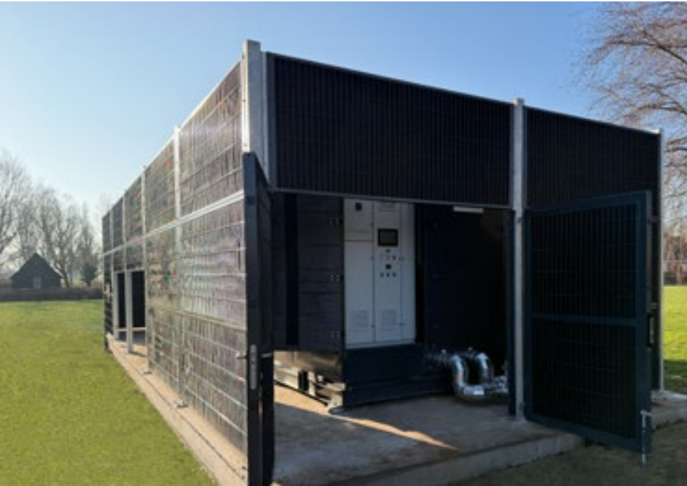
The heat pump is enclosed by sound panels.
