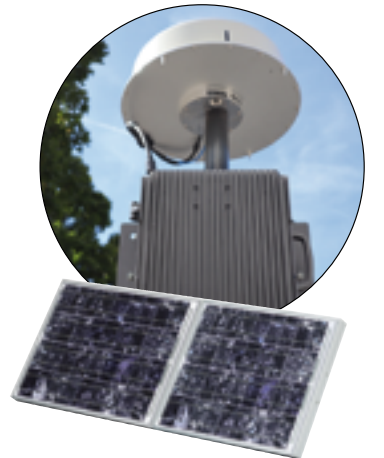
Mast mounted Outdoor Unit with solar panel
