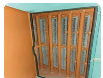
Clean gas-side installation Horizontal
