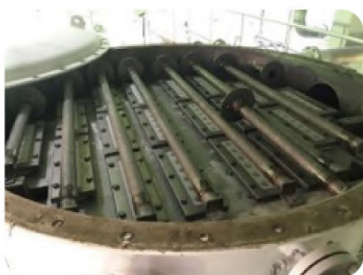
Clean gas-side installation Vertical
