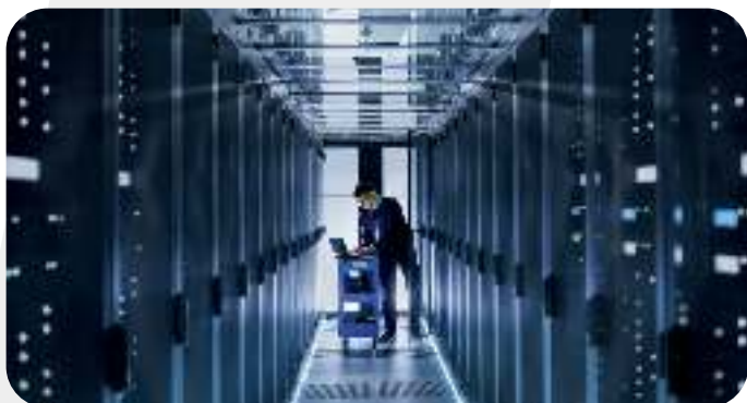
DATA CENTRE ECMWF
