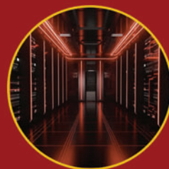
Cloud & Data Center
