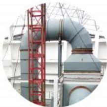
Energy Saving & Emission Reduction (Low-temperature Waste Heat)
