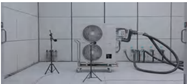
05 A/C Noise & Vibration Lab: 6 semi-anechoic chambers
