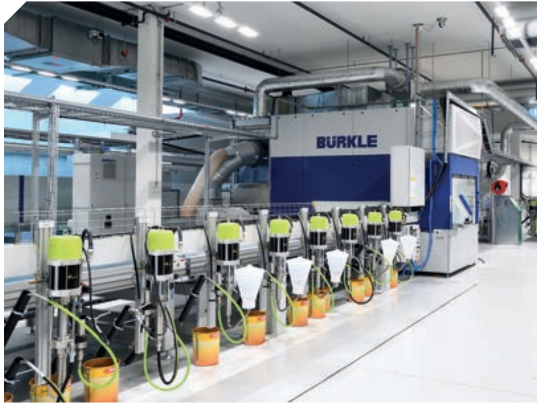
High-performance spray coating line with flexible color change system.
