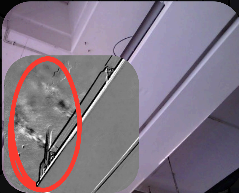
Detection on evaporator from approx. 7 m distance
