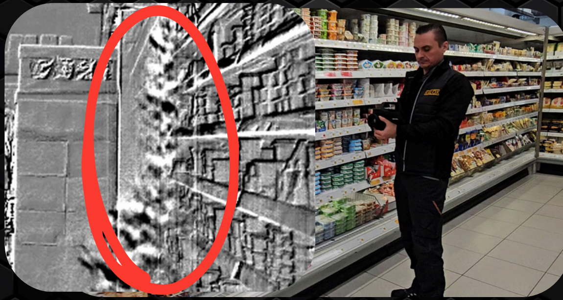
Detection on refrigerated wall cabinet during operation
