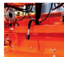
Battery charging cable
