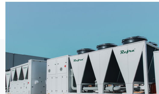
How Refra Propane Heat Pump and Chiller Keep 5 Million Bouquets Fresh in Ireland
