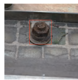
Metal Corrosion Segmentation
