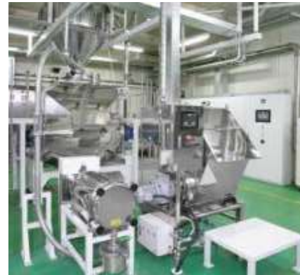
5. Equipment for in-feeding and conveying supplemental materials
