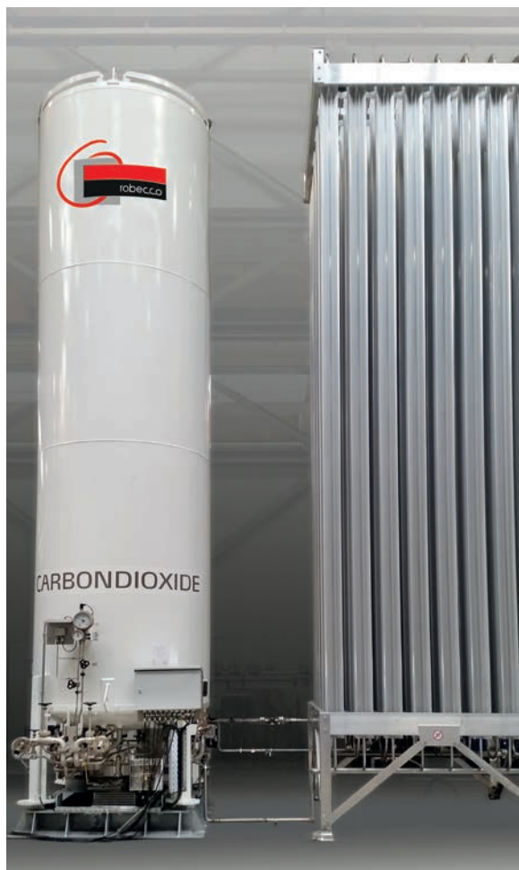
Figure 1. CO 2 low-pressure tank with ambient evaporiser.
