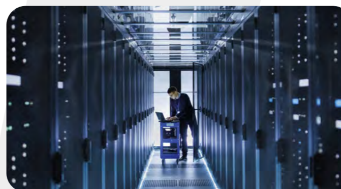
DATA CENTRE ECMWF Bologna - Italy
