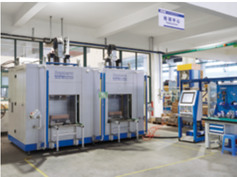
BPHE Helium Leakage Detector
